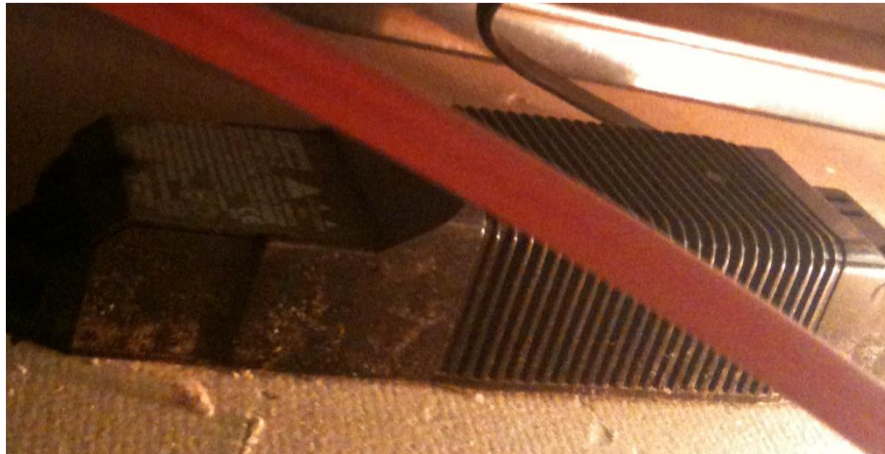
Figure 5: Magnetic transformer in ceiling space
