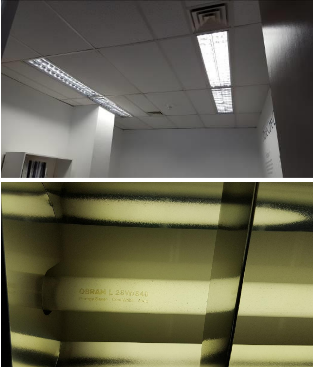
Figure 26: Photographs showing the twin tube 28W T5 HE luminaires
