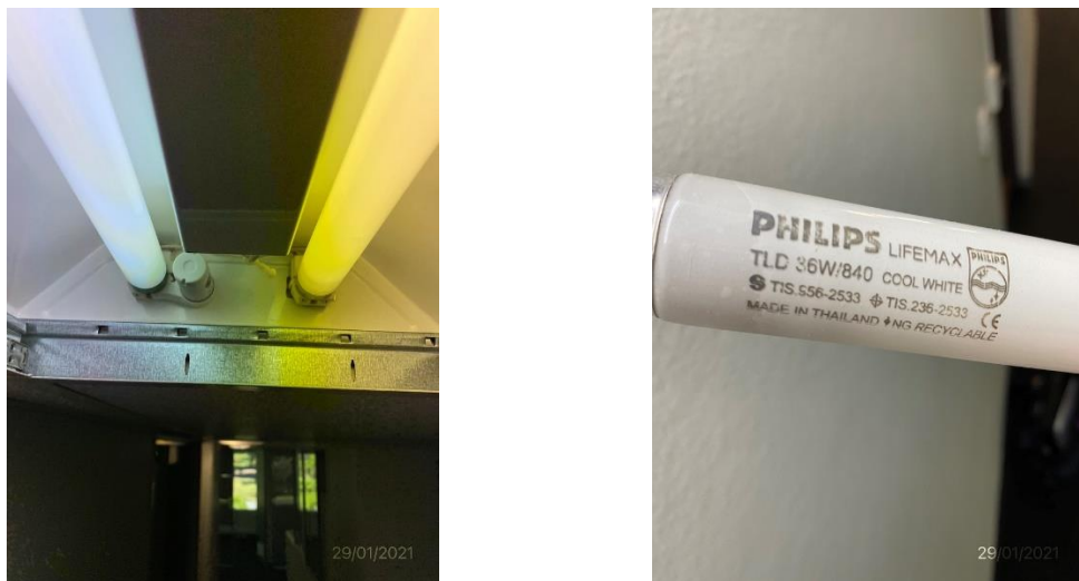
Figure 22: Photographs showing 2x36W T8 fluorescent tubes.
